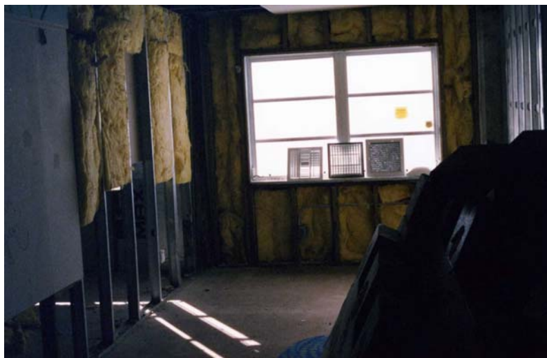
Children's Advocacy Center, Naples, FL following Hurricane Wilma October 24, 2005
